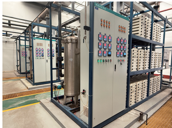
Figure 5-9 Risun China Gas Water Resource Control Equipment
