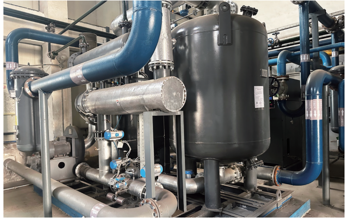
Figure 5-4 Dryer "One in operation and one on standby"
