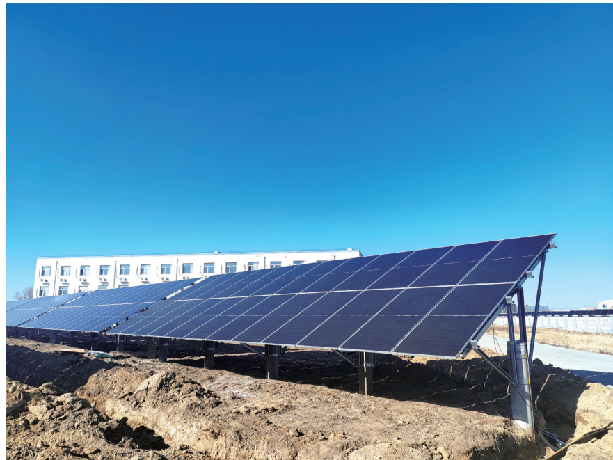
Figure 5-5 Photovoltaic Equipment at the Group's Laoting Base
